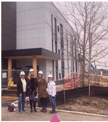
Construction begins on Block Line Affordable Housing for 10 women and their children
